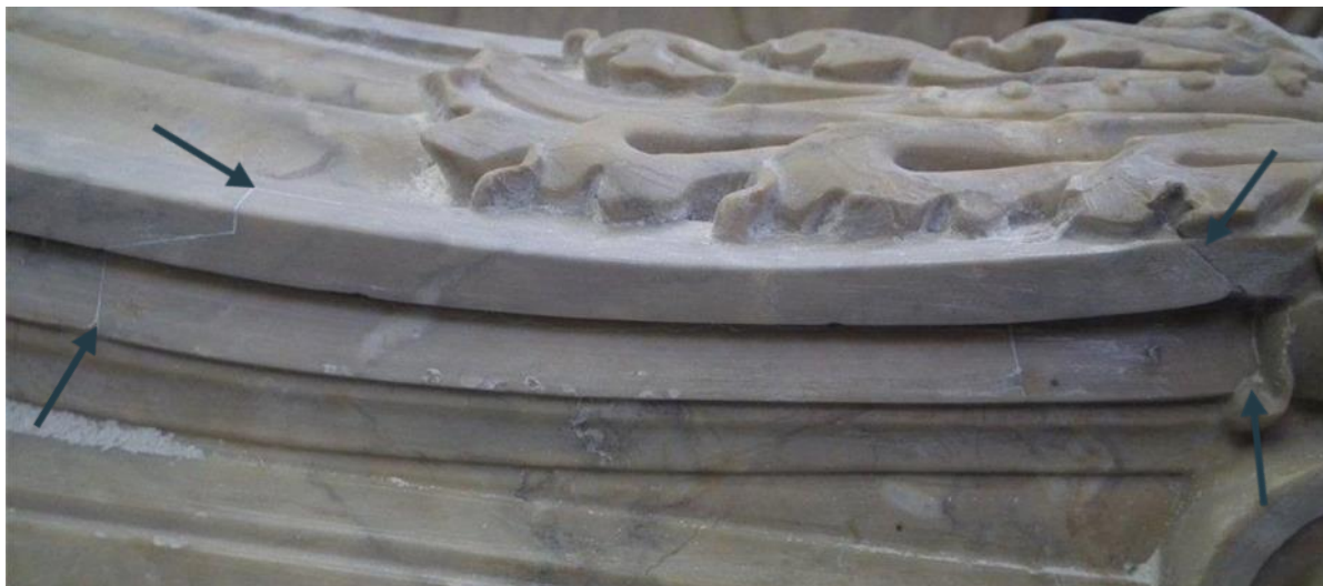
Plate 9: Detail of the outer edge of a left hand jamb. A new section of repair has been let into the original, the joint line only being visible during cleaning work, as indicated by the arrows on the image above. The process can be seen to illustrate the savings incurred by minimalizing wastage of the block.
