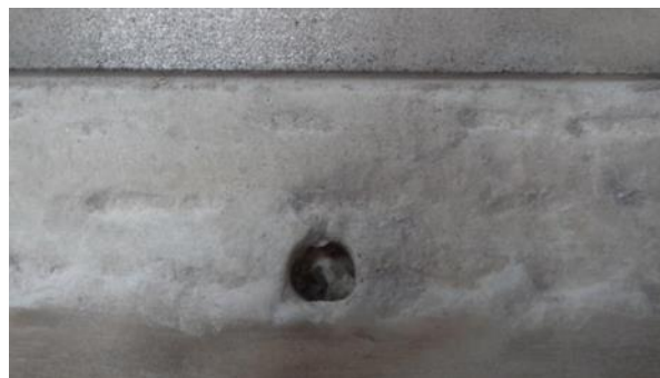
Plate 7: Detail looking down onto the top face of the soffit, showing the hole to the centre of the soffit, almost certainly intended to allow for the introduction of a bolt to support the underside of the soffit, but never introduced. The sheen to the top seen face of the soffit bears comparison to the chiselled unseen side, with the sheen of the former a result of acid cleaning in the past.
